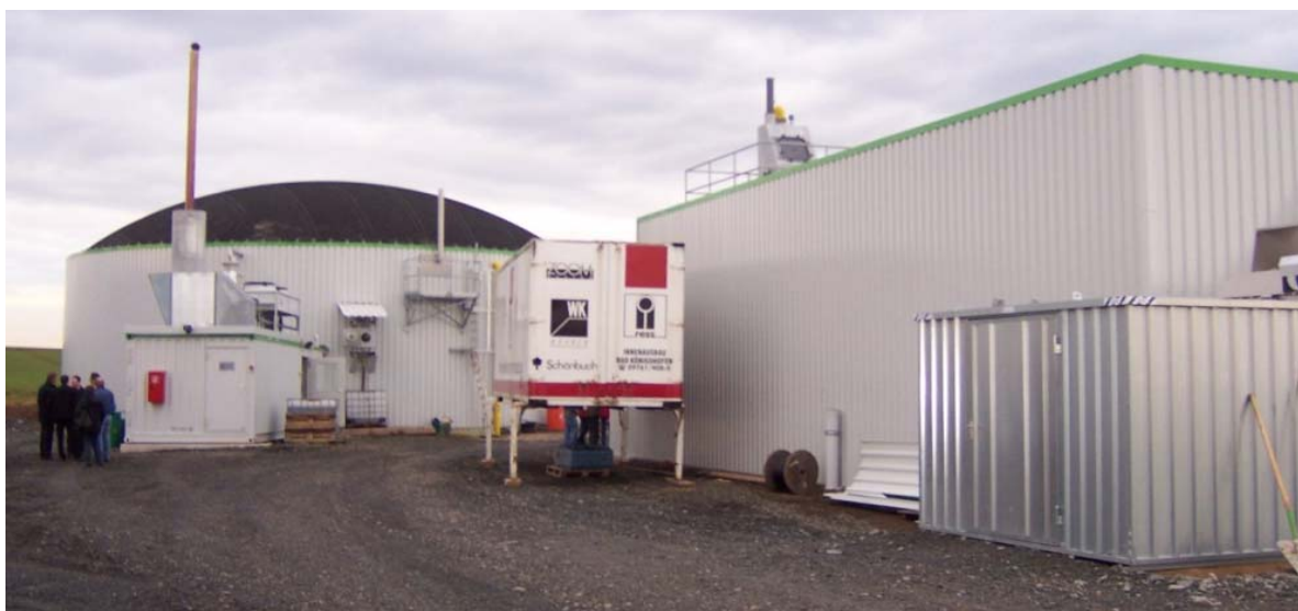
Figure 35: Biogas installation with two digesters (continuously flow type on the left and pug flow type container on the right) in Germany
